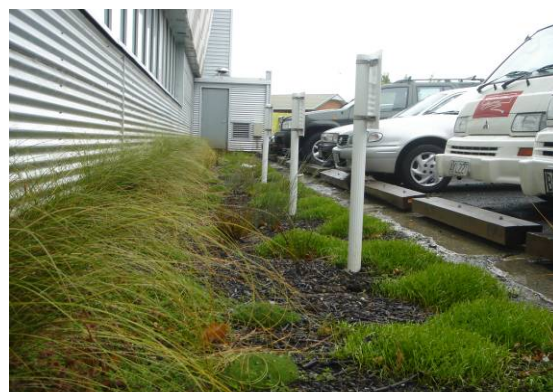
(Right) Bioretention swale, Landcare Research, Auckland, with Carex against the building and Libertia, Scleranthus biflorus, Selliera radicans, Pratia, and Acaena. Note the lack of curb allows water to run off from carpark. Photo: Robyn Simcock
