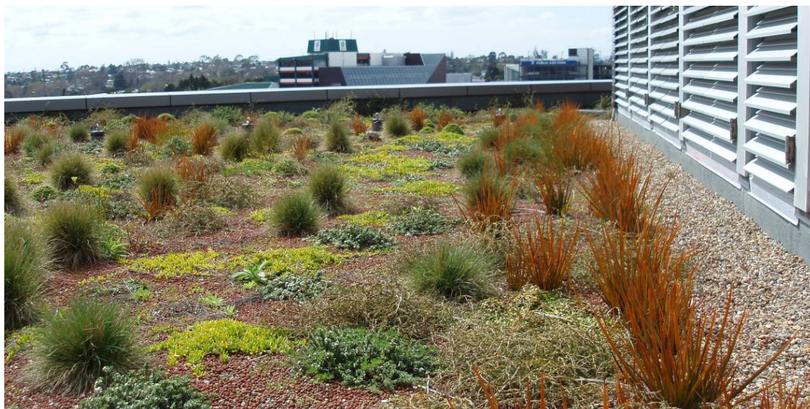
Figure 21 Waitakere Civic Centre, semi-extensive green roof at about 16 months old. Photo: Robyn Simcock
