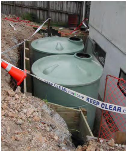
Figure 22: Rain water tanks installed at Glencourt Place Photo: Eva Veseley
