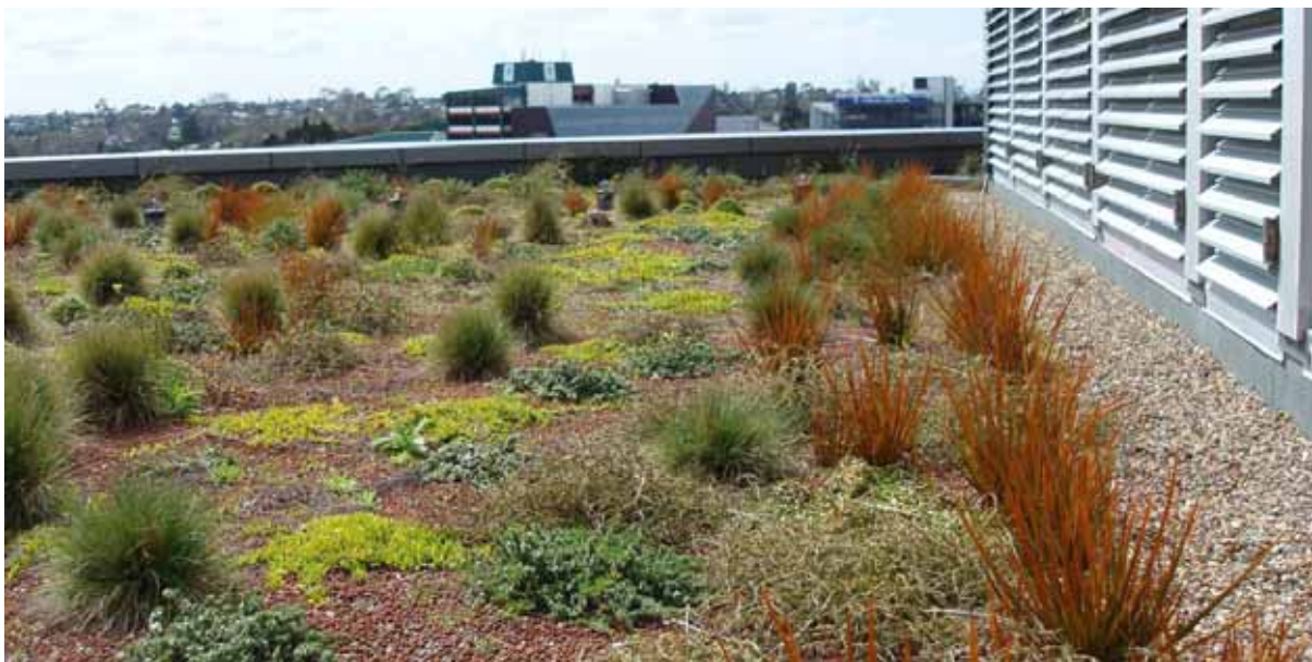
Figure 20: Waitakere Civic Centre (New Zealand) extensive green roof at about 16 months old. Extensive roofs are generally self-watering from rainfall. Photo: Robyn Simcock
