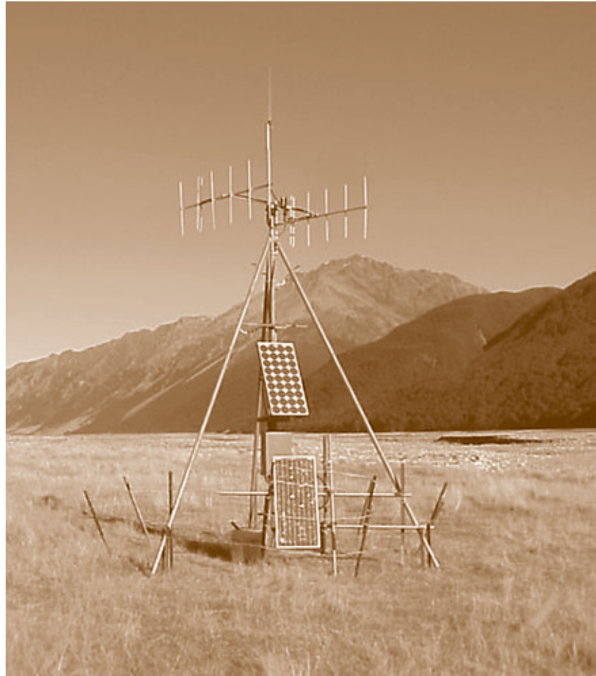
One tower of the new system, including, from the top, a whip radio aerial and double yagi (that feed into the dual receiver), UHF whip aerial, solar panel, electronic control unit, a second solar panel (for additional charging), and heavy-duty batteries.
