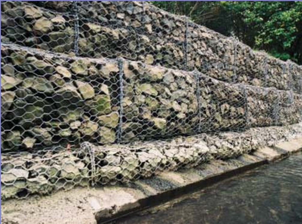
Gabion blocks help prevent land slippage caused by erosion. (Meola Creek).
