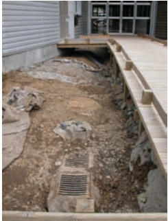
The site unmasked prior to raingarden construction, revealing infrastructure to be avoided: two stormwater grates, a manhole cover (sewage) and outlet to the stormwater system.
