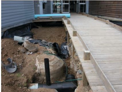
Excavation complete and subsoil in place. Rock underlies the site, limiting excavation depth. We decided to avoid the infrastructure and only fully excavate the irrigated area to 1.1m depth. Iron oxides give the subsoil its nut-brown colour. The black plastic lining can be seen protecting the building foundations and at the front of the raingarden. The blue pipe will be connected to the horizontal black pipe which discharges to the Auckland University stormwater system.
