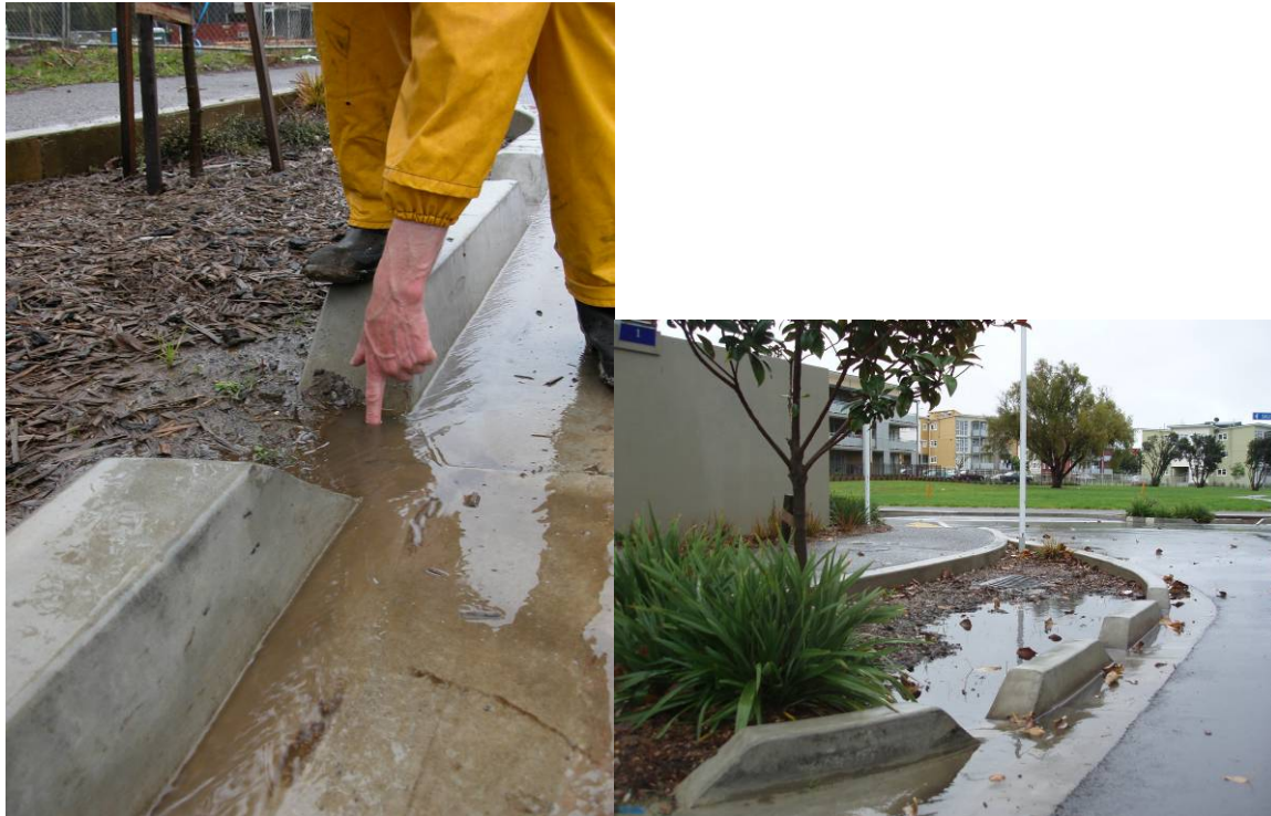
During construction of houses, sediment eroded from the building sites was captured in some rain gardens until it prevented water flowing into the rain gardens (left photo, July 2006). Most rain gardens were constructed with less than the specified 220 mm ponding depth, generally due to a combination of overfilling of the raingarden with soil and mulch, and the overflow grates being set too low. This means in places stormwater can short-circuit the raingarden, reducing treatment efficiency and volume detained (photo July 2007)
