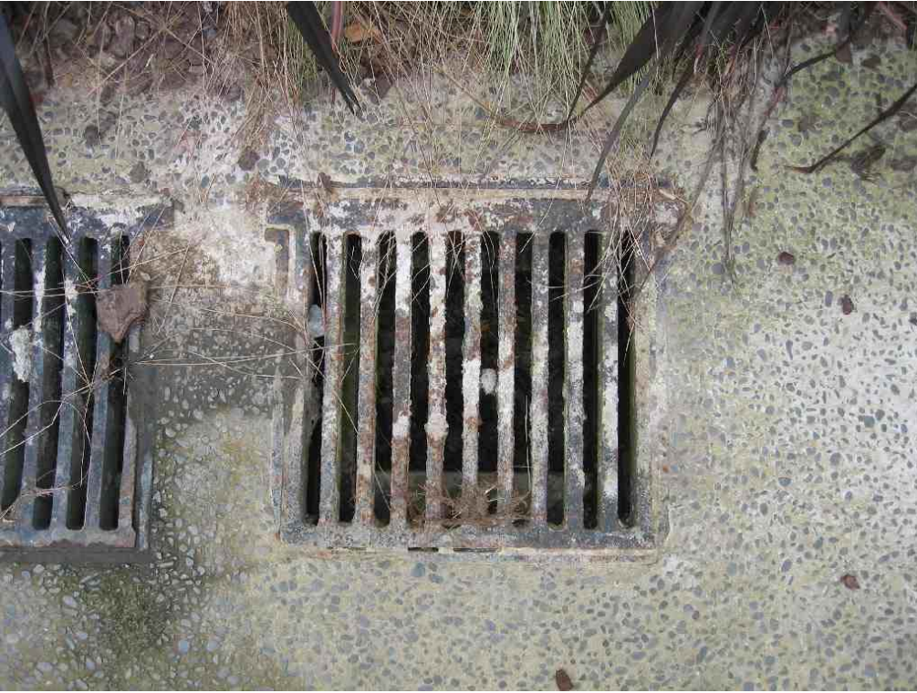
Photograph 2: Catch-pit inserts for paved-area runoff at Tiritiri Road
