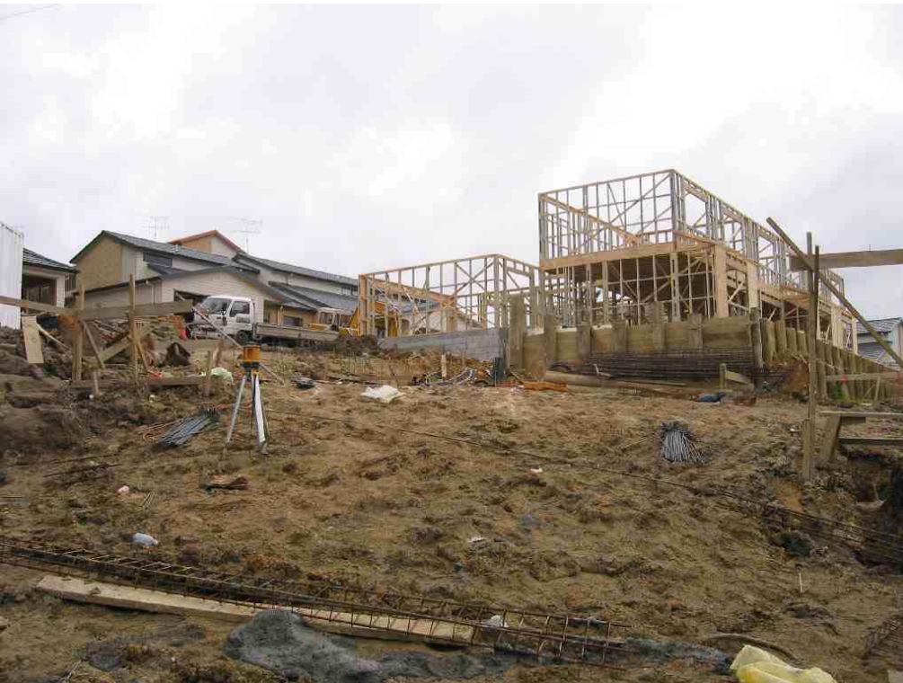
Photograph 7: Serious site runoff during construction at Verbena Road
