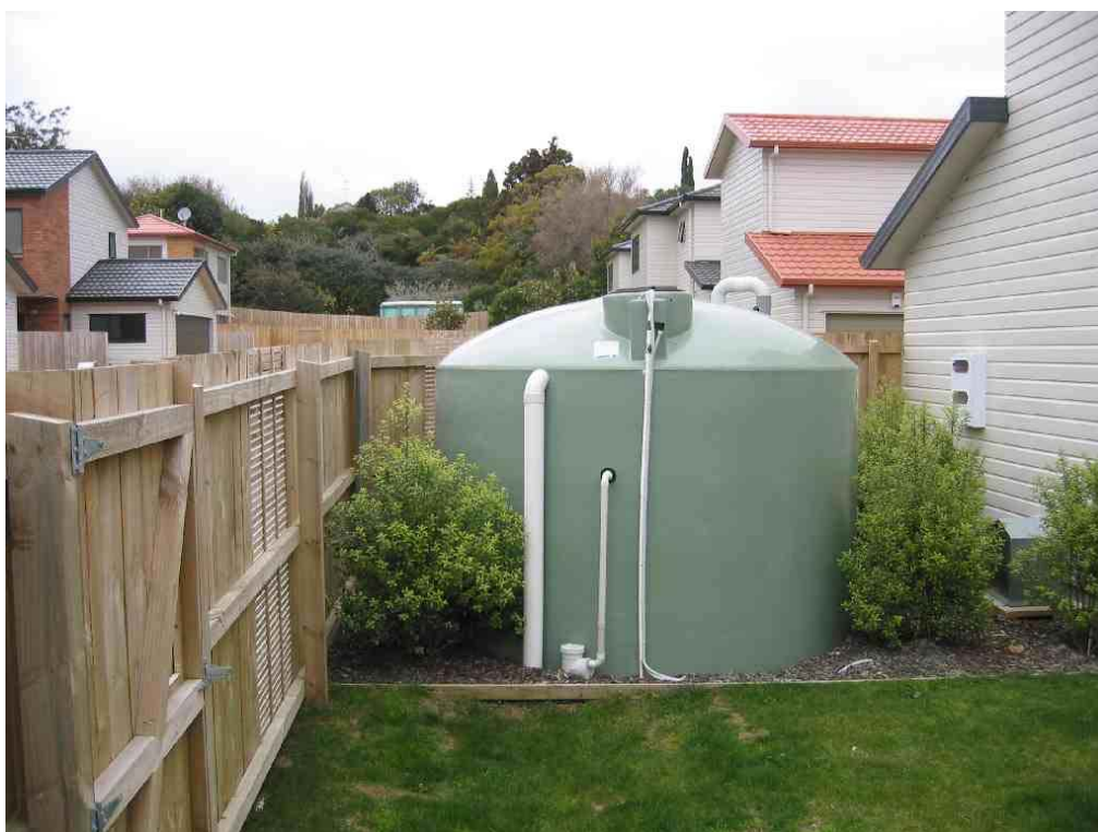
Photograph 1: Rain tank for roof-water collection for re-use at Tiritiri Road
