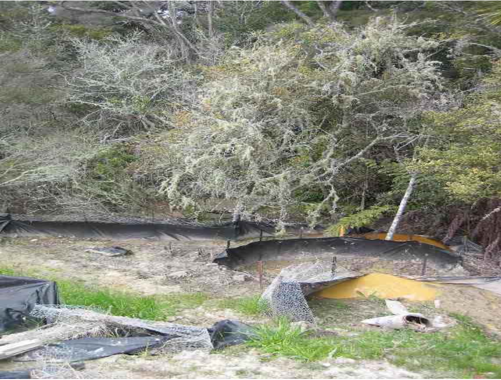
Photograph 8: Visible damage at Verbena Road during construction
