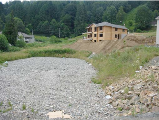
Photograph 3 Chilliwack, Vancouver, stormwater infiltration gallery
