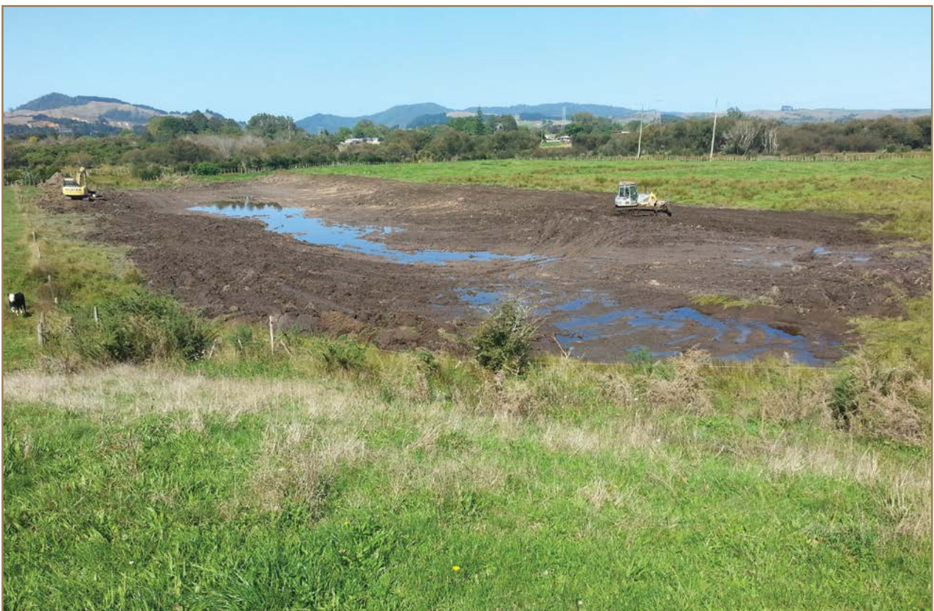
Diggers preparing one of the tuna ponds, Raahui Pookeka. Photo: Erina Watene-Rawiri
