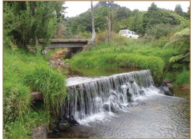
Waiharakeke Stream ford, Utakura River catchment, Northland. The ford is 1.5m high and restricts the ability of eels to reach habitats upstream. Photo: © NIWA
