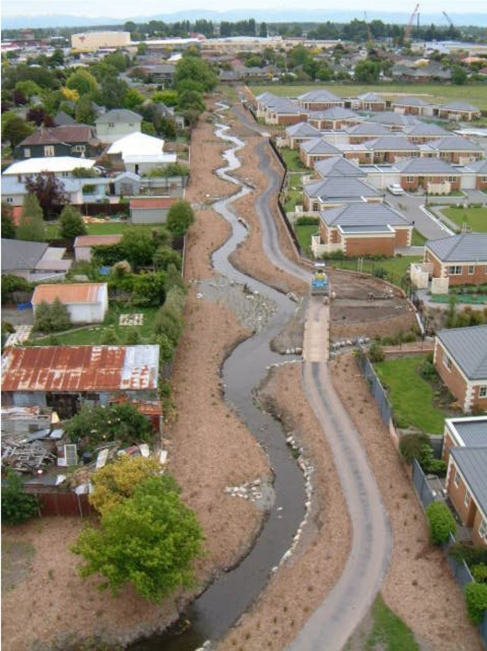
Papanui Stream under construction: a transformation from a timber-sided utility drain to a stream formed with meanders, pools, riffles and runs along with logs and rocks to provide a diverse aquatic habitat. This was a collaborative, multidisciplinary project (CCC NPGU)
