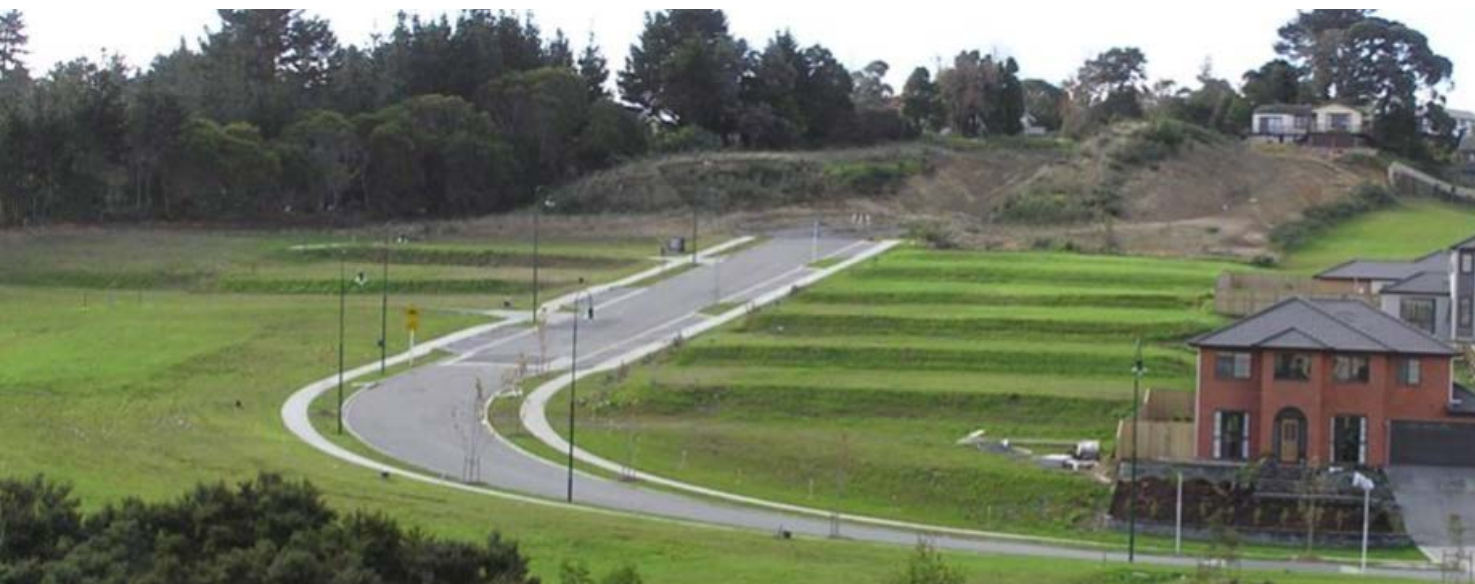
Terracing and land contouring creates flat, geotechnically stable land for establishing roads and concrete foundations.
