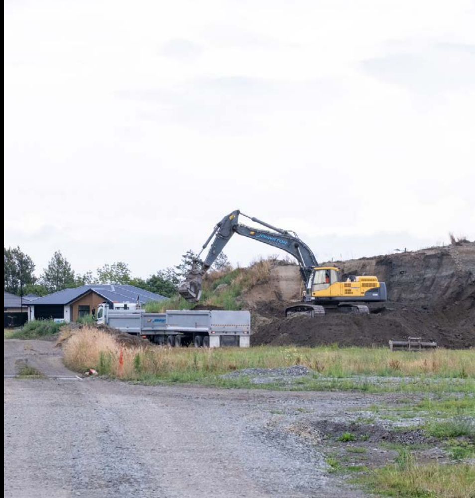
Housing developments create huge disturbances of soil, often leaving quantities of unwanted or surplus soil.
