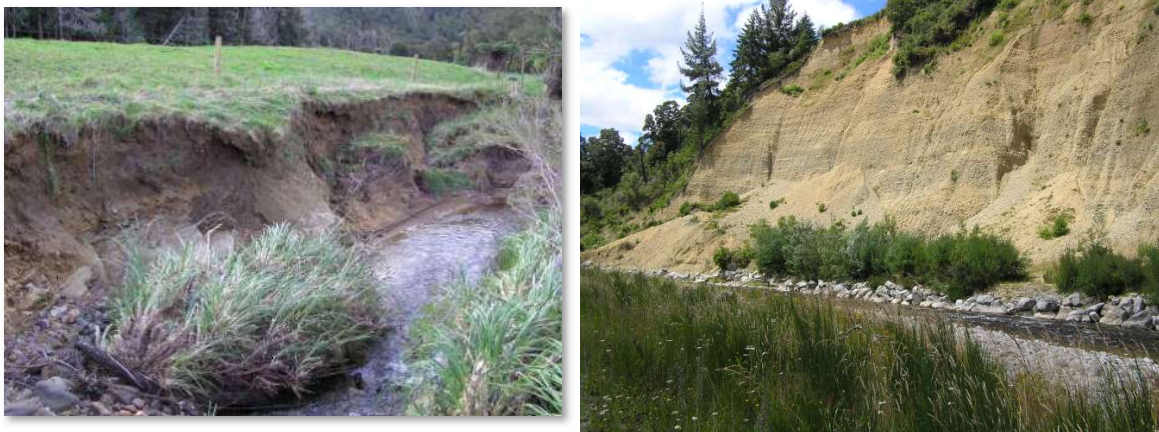
Figure 6. Examples of streambank erosion.
